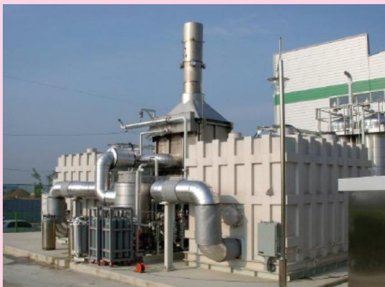
Figure 8 FCE's 2.8MW DFC3000 installed in Korea
