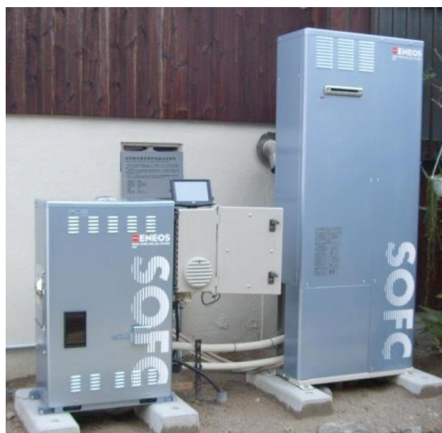
Figure 2: Nippon Oil SOFC, 0.7kW fuel cell unit on the left hand side, hot water tank unit on the right hand side.
