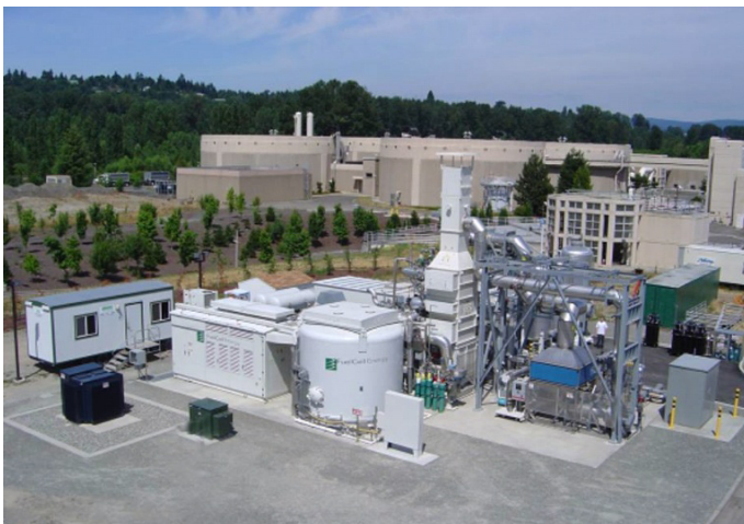
Figure 2. King County Power Plant (courtesy of FCE)
