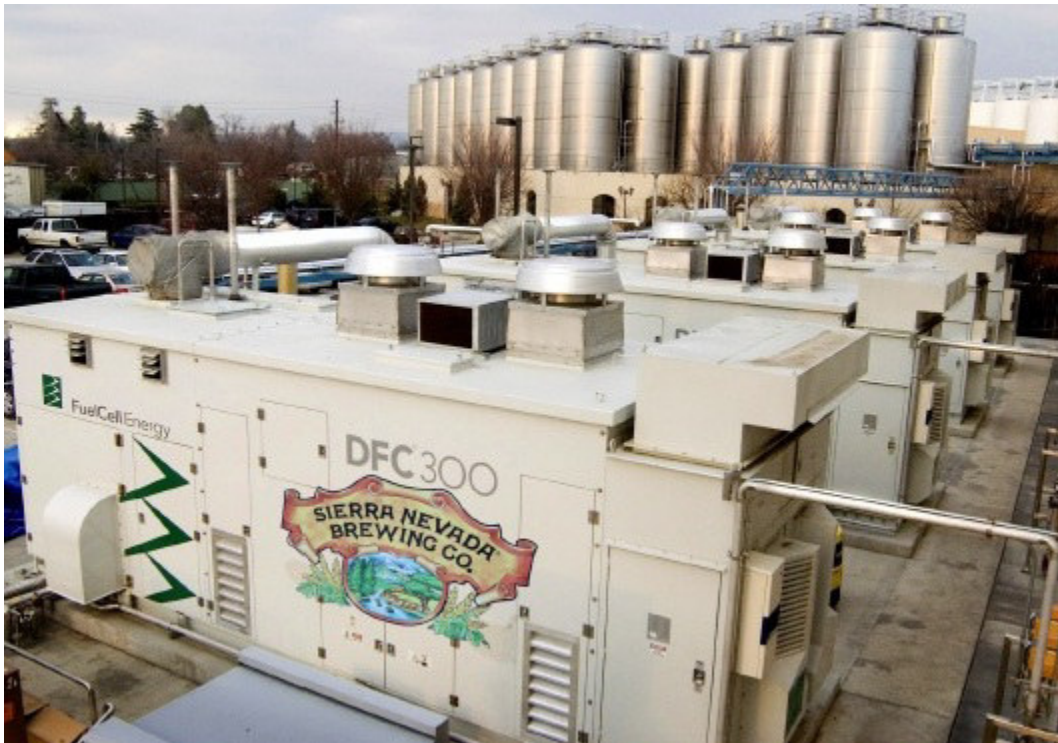
FIGURE 225 A view of the four DFC300 system by Fuelcell Energy at Sierra Nevada brewery 9
