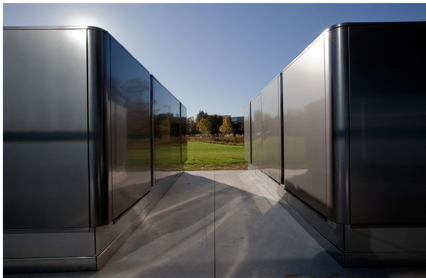
FIGURE 156 Apple 10 MW SOFC farm made up of 50 Bloom Energy boxes rated 200kW each in Conover, North Carolina 4
