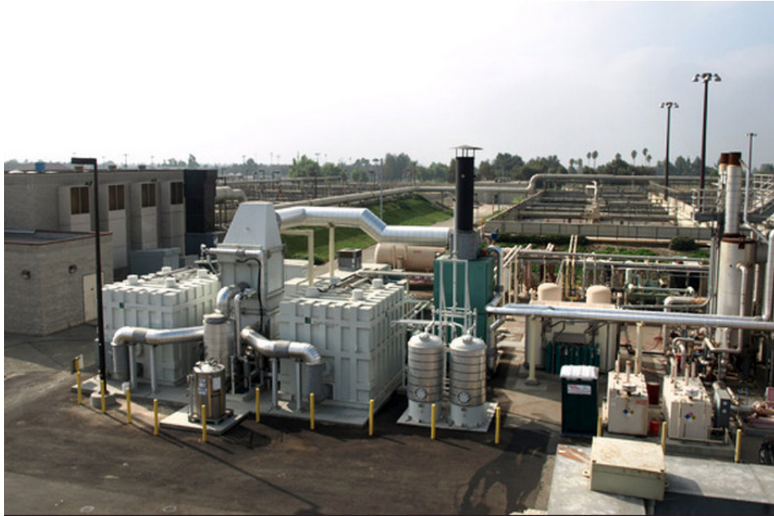
FIGURE 214 IEUA regional wastewater treatment plant 1 (RP-1)
