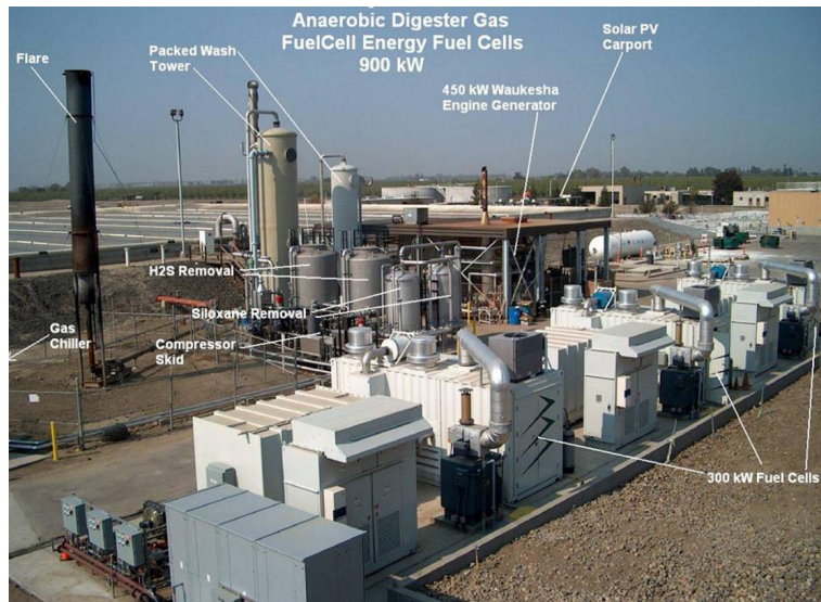
FIGURE 247 Original installation of Three FuelCell Energy Fuel Cells and Gas Pretreatment Unit at Tulare Wastewater Treatment Plant
