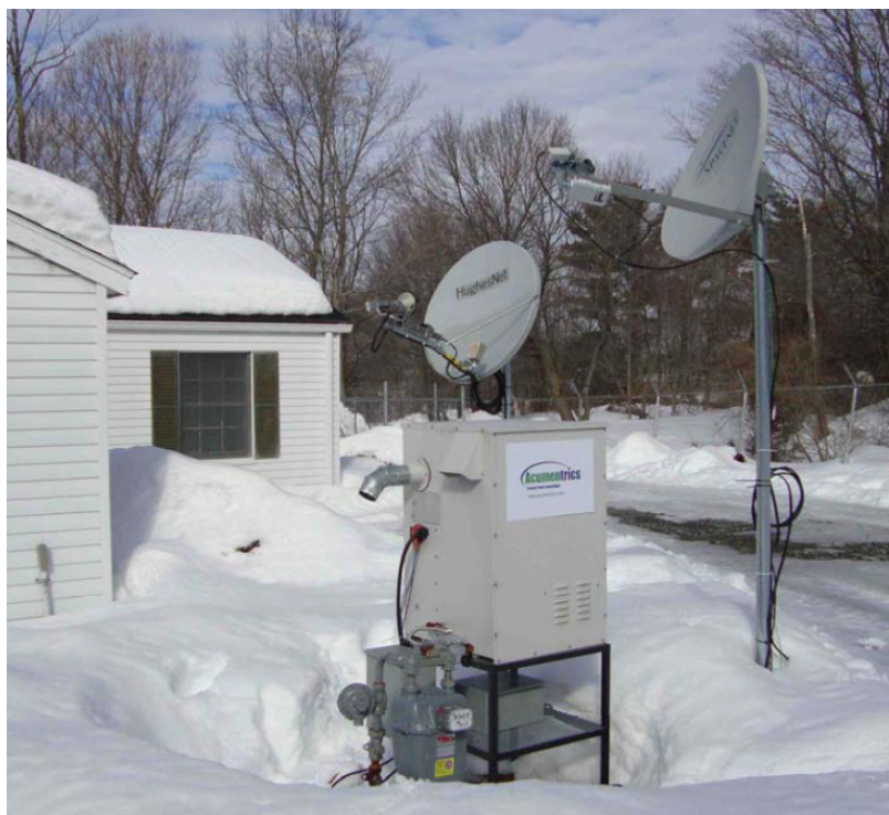
Figure 12. An example of remote, stand-alone power supply.
