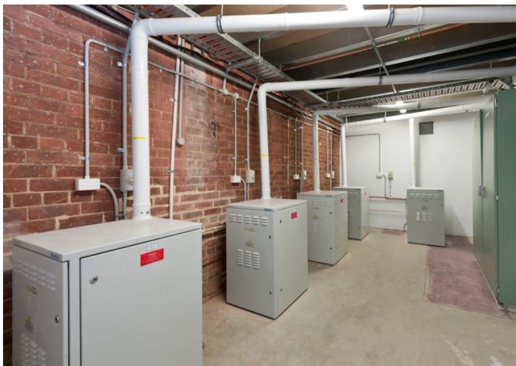
Figure 46. BlueGens installed in March 2012 as retrofit of a Commercial building in Adelaide (over 7 tonnes of carbon saved in first 3 months). [source: CFCL, Clean Power for Global Markets Shareholder Update 2012 ]
