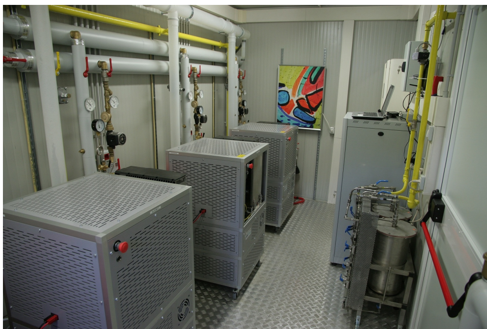
Figure 36. "Isola Cogenerativa" is the first SOFC cogeneration plant in Italy; it consists of 3 modules of 1 kW el fueled by natural gas, for a total of 3 kW of electricity and 6 kW of heat for domestic hot water.
